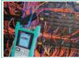
Fiber optic power test
