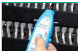
STP wire tracing
