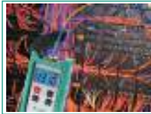
Fiber optic power test
