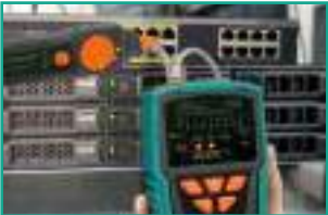
PoE switches & wire tracing
