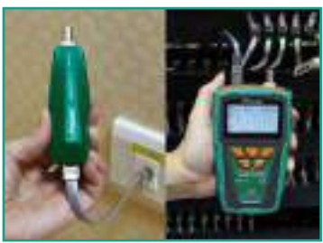
Verify LAN/ Telephone /Coaxial cable condition
